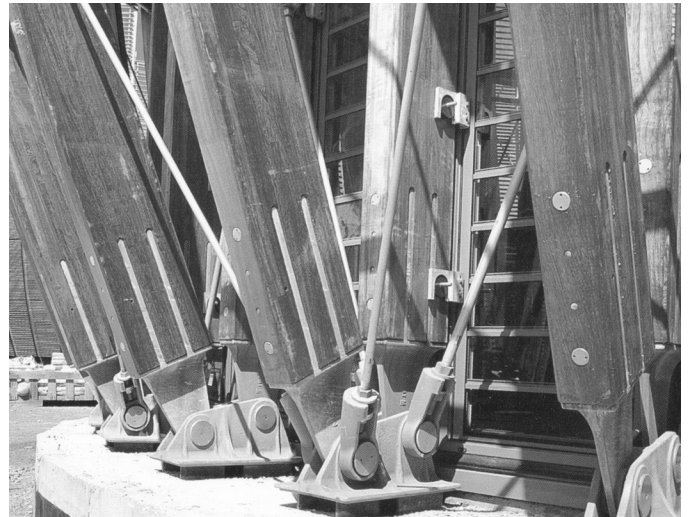
Fig. 5. Case Detail of Jean-Marie Tjibaou Cultural Center. Courtesy of Renzo Piano Building Workshop.
